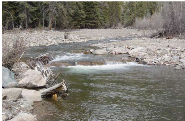
Figure 11-31 Cross vane/rootwad/log vane step-pool, converting a braided D4→C4 stream type on the East Fork Piedra River, CO
